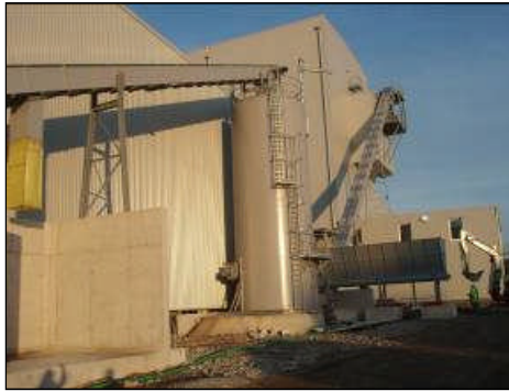
13 Figure 2: Conveyor for wood chips from timber silo
